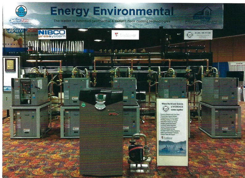
This 1.5 million BTU/hr hybrid vapor injection heat pump and boiler system for an Aspen home delivers superior comfort using hydronic heating or cooling, DHW, snowmelt, and pool heating at four times the efficiency of a conventional system. (IGSHPA Conference)
